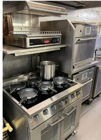
Electric kitchen equipment
